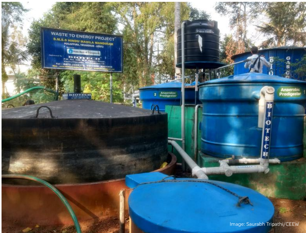
FIGURE 10: Community biogas plant
